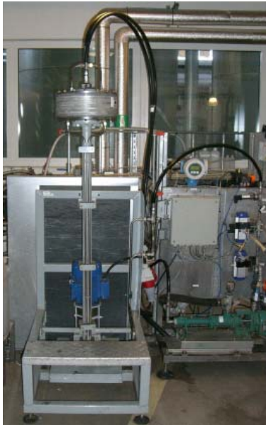
Figure 11: VSEP unit (membrane stack and electrical engine) 1 .
